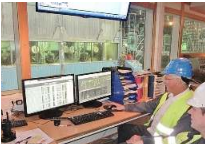
Fig. 10: Control via process leading system
