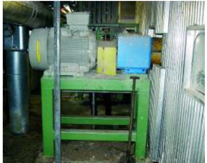
Fig. 1: Standard motor with pre-gear and console outside of the hood
