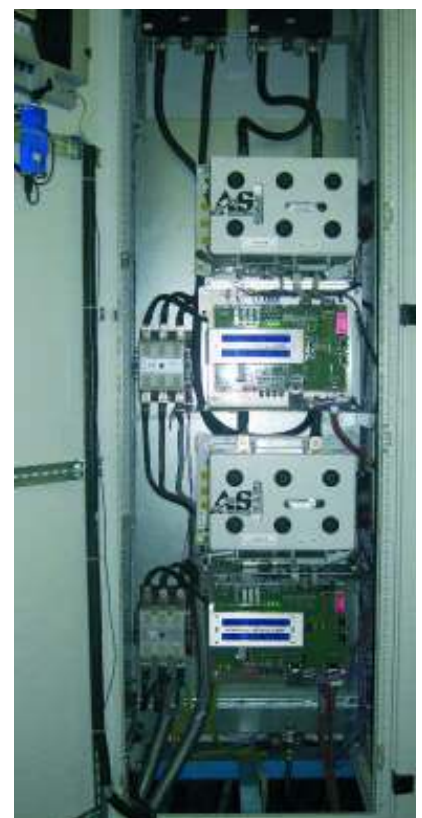
Fig. 6: View inside the cabinet with the frequency converter FlexoDynamic
